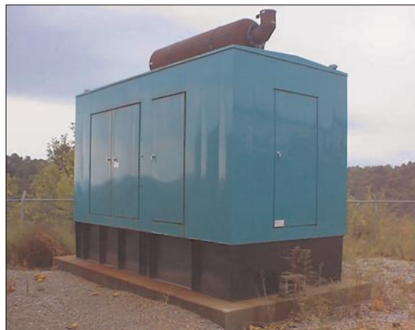
A larger 800 kW Generator.
