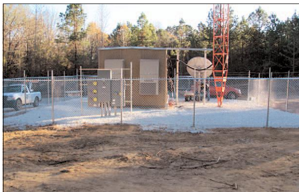
KLHV's transmitter site. All were products supplied by Jampro.
