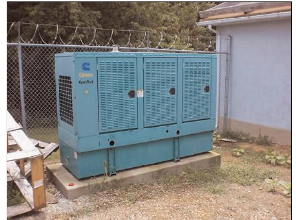
A modest-sized generator for broadcast use.
