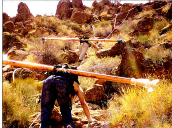
Interbay feed lines being carried up the slope, that in places was up to a 75 degree angle.
