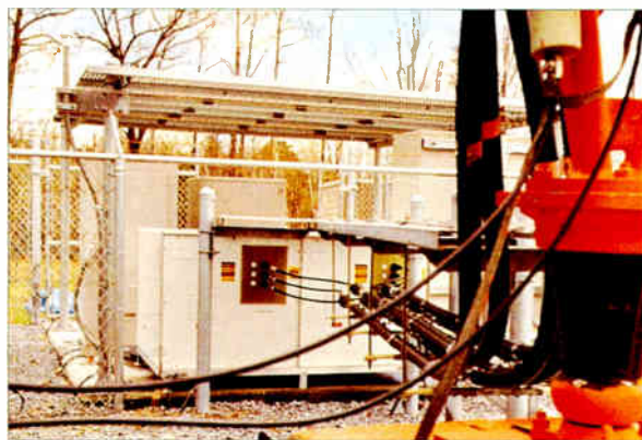
CoLoCoils® at WJOY in Burlington, VT
