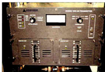
CFRX's Armstrong X1000B SW transmitter installed.
