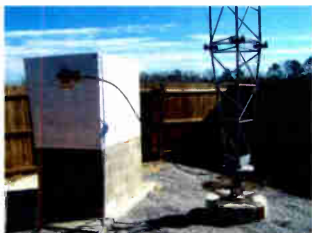
High-Power Antenna Tuning Units
