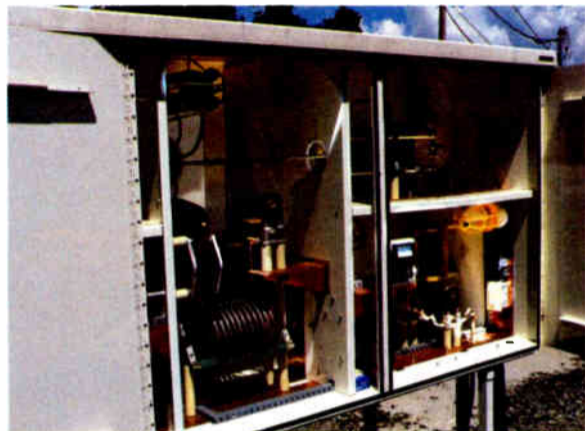
Part of an installed combiner cabinet.
