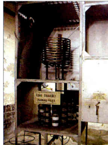
The WLW second harmonic filter today. The switch on the right selected 50 or 500 kW operation.
