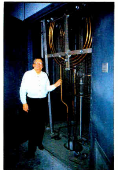
Clyde Haehnle at the rear of a power amplifier output cubicle.
