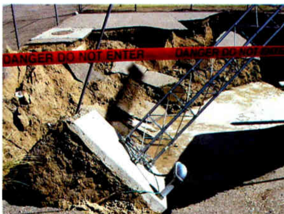
Still attached to the base, but not at the right angle.
