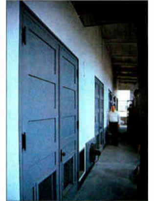
The rear doors of the WLW 500 KW transmitter.
