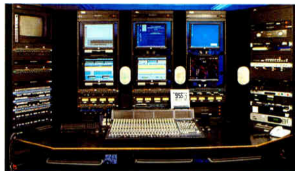
The comprehensive BSI installation at GAB.
