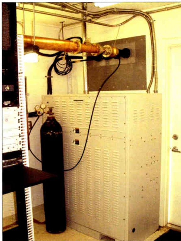
Would you be satisfied with this installation?
