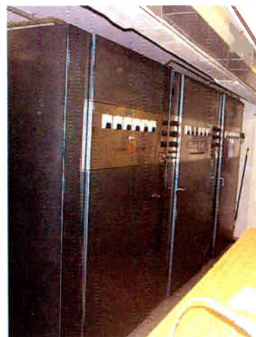
One of the last AM transmitters built by GE, the BT-50C.
