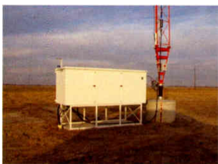
The ATU for Tower 1 was finally in place on its concrete slab, ready for testing.
