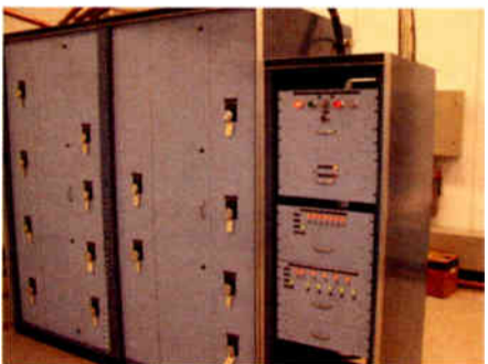
A custom control system provides for three modes of regular operation.
