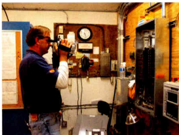
Mike Bivens of Infrared Services, Inc. views the breaker box with an infrared camera.
