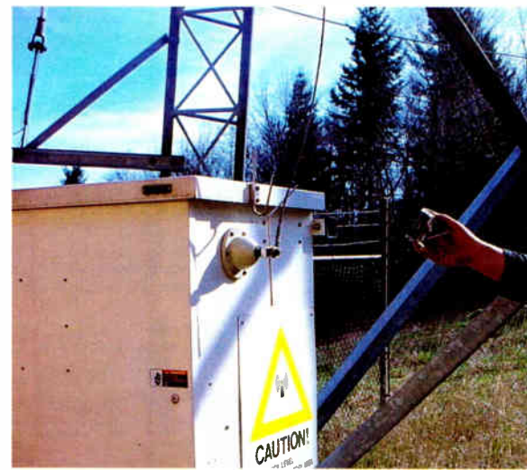
Detuning box at a communications tower.
