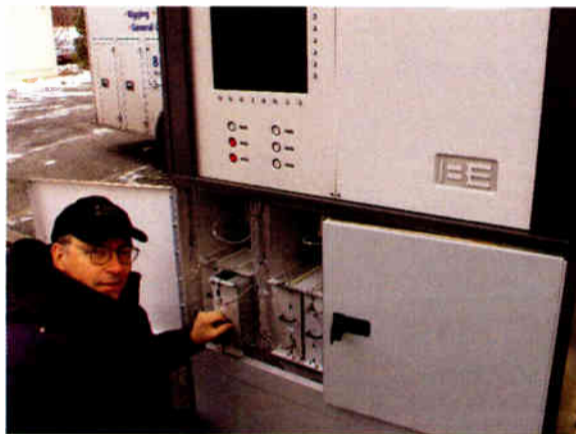
Loud & Clean's John Garrett tags and removes all the RF Power Supply and PA modules to lighten the 4MX 50 cabinet for insertion into the room.
