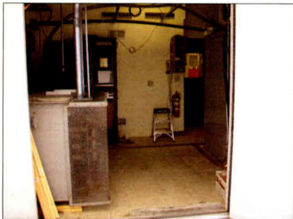
If WBIX was to get a new 50 kW transmitter, it had to go here.
