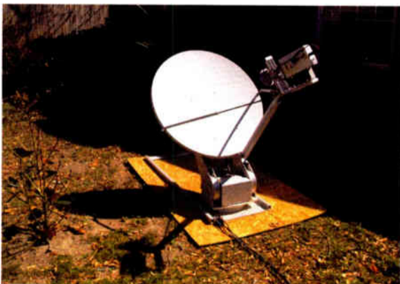
Crews quickly installed satellite downlinks to connect the stations with the outside world, both for communications and program channels.
