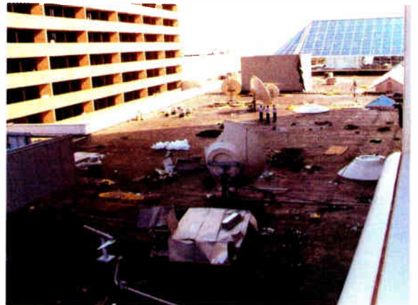
The various satellite dishes did not fare so well in the hurricane. (Note the dishes laying on the roof and the one with the giant "bite" take by Katrina.)
