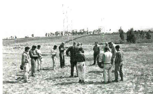
Getting ready for the erection. The shorter towers are vertical, the 240 foot sticks are laying on the ground. (The author is just left of the left tower.)
