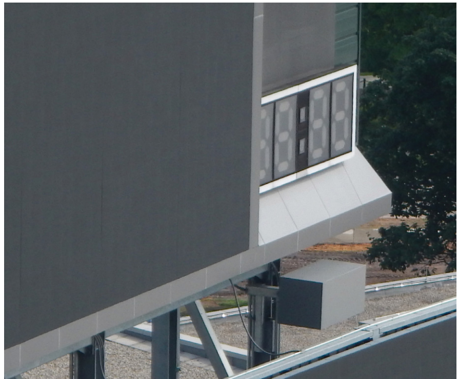
The gray box made of RF-friendly materials and mounted below the digital time display houses antennas for the distributed antenna system in Spartan Stadium.
