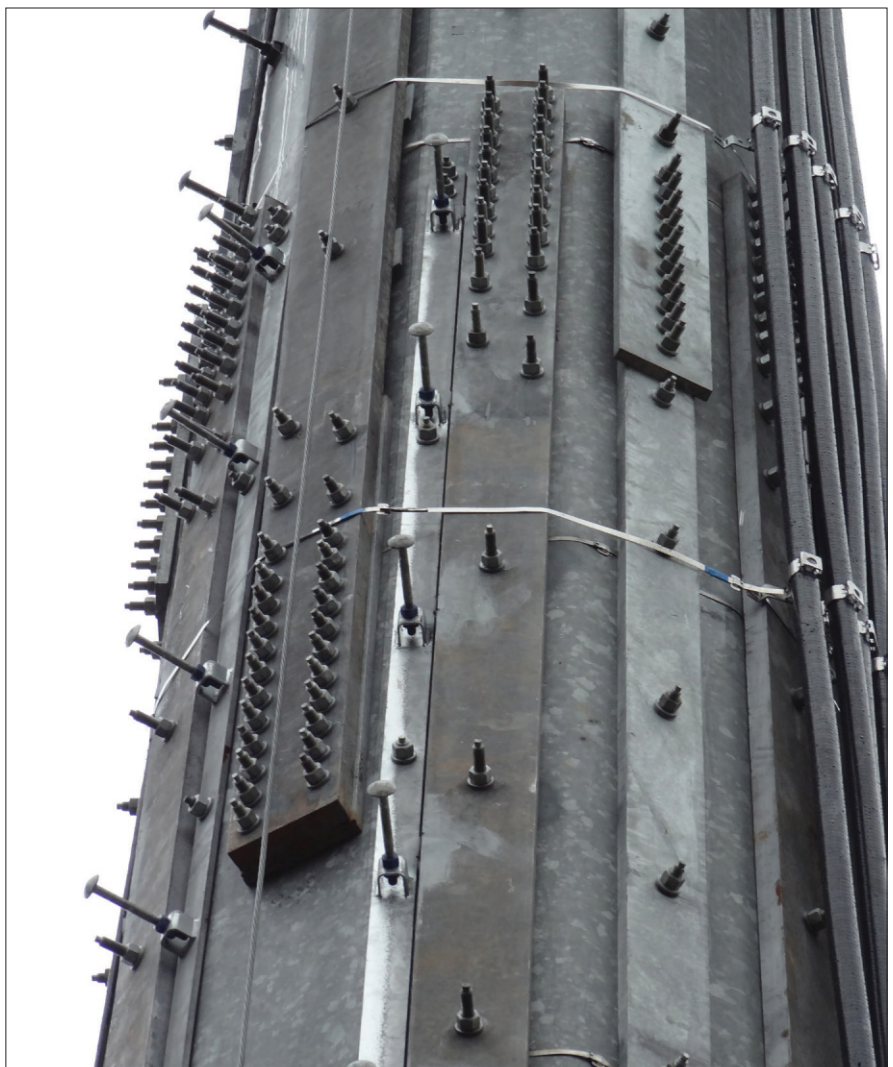
Photo 1. A heavily reinforced monopole.
