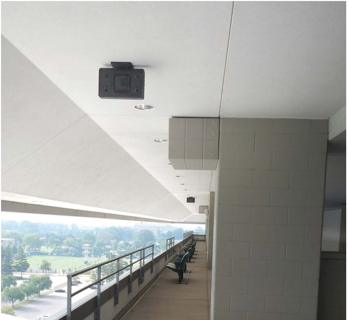
Part of a suite of concealment systems delivered by Stealth Concealment Solutions, a distributed antenna system antenna enclosure hangs from the ceiling in an area of the Spartan Stadium.
