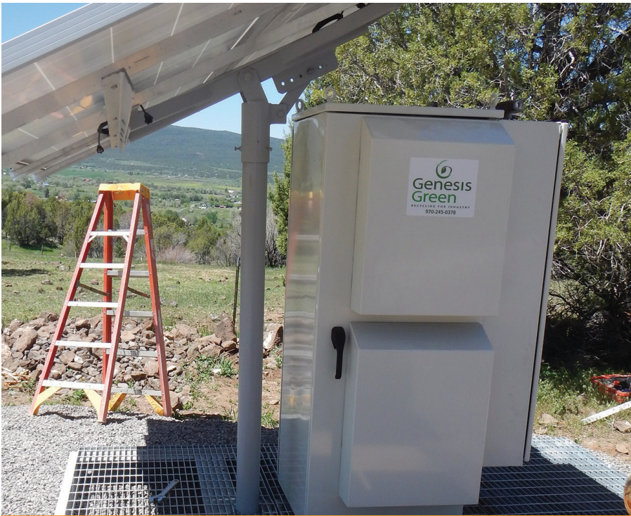
The reuse of battery and power cabinets for solar power may not have any applications for cell sites, but it might find a home in the oil and gas industry. Photo courtesy of Teltech Communications
