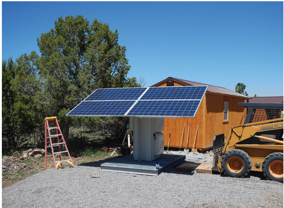
Teltech Communications' first solar prototype repurposes battery and power cabinets. Photo courtesy of Teltech Communications
