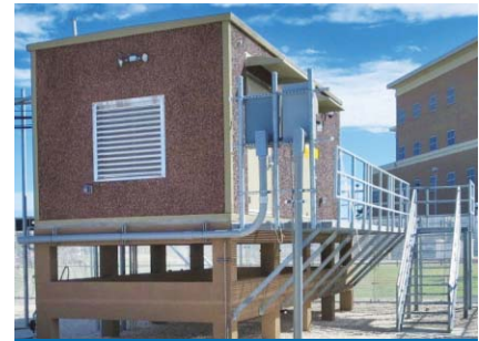
The Galveston County Emergency Communications District installation includes stairs and a grate alongside the shelter for access to the elevated shelter doors.
