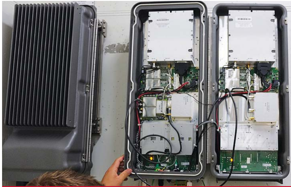
A remote unit in a communications equipment room.
