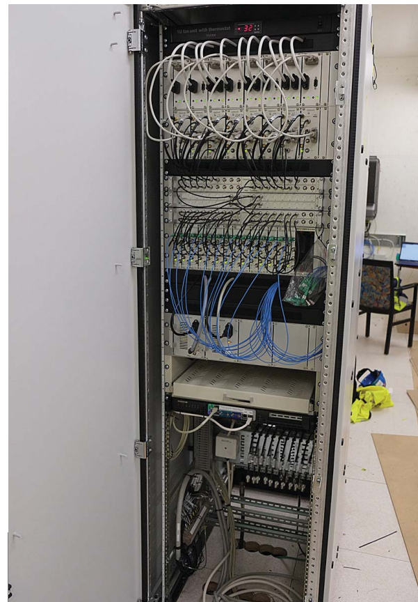
A distributed antenna system (DAS) in a communications equipment room.
