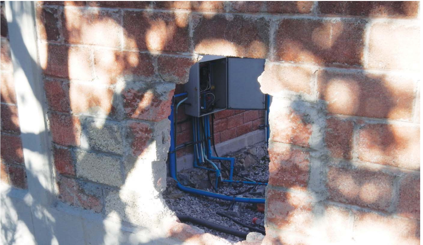
From evidence of previous repair, it looks as though this wall has been penetrated more than once by thieves who avoid the shelter door and use brute force to enter the equipment building. Photo courtesy of Westell Technologies
