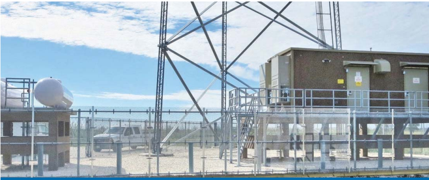
Consolidated Telecom Services used a Kenner chain wall system to elevate a communications equipment shelter and propane tanks in Galveston County, Texas, in August 2013.
