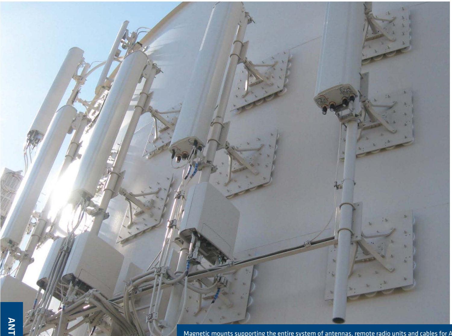
Magnetic mounts supporting the entire system of antennas, remote radio units and cables for AT&T. Photography by Tai Irish, Goodman Networks.
