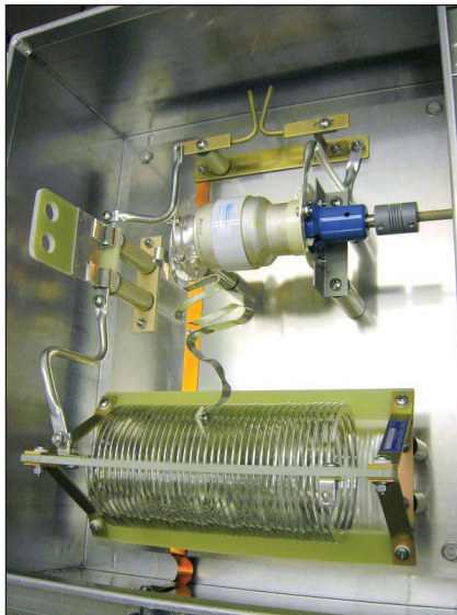
A capacitor (top) and inductor form a network that tunes the tower skirt to make the tower nonresonant at the AM station frequency. Photo courtesy of Waterford Consultants/Larry Giessman
