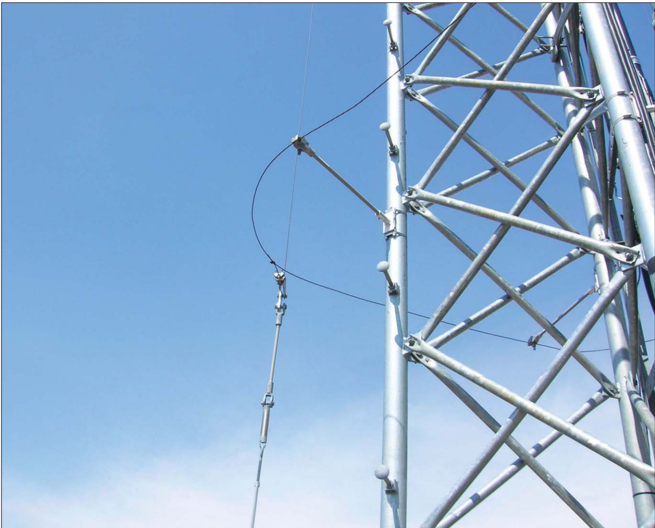
Stand-off insulators support a portion of the wire skirt engineered specifically for the cellular tower. Photo courtesy of Waterford Consultants/Larry Giessman
