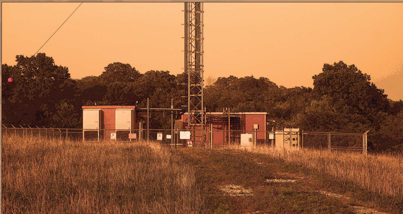
Among tower owners, taking ownership of the land beneath their towers is becoming increasingly important.
