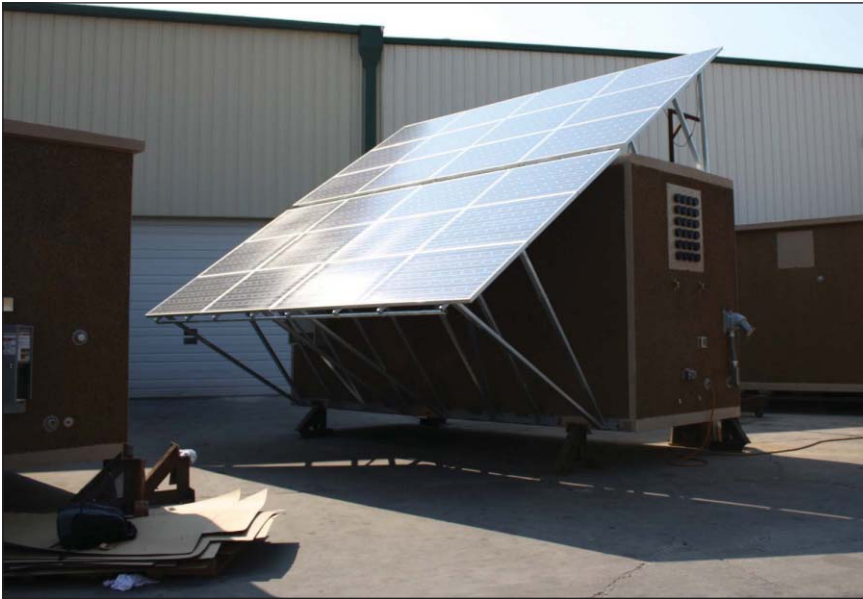
A solar array attached to an equipment shelter for deployment at a California site.
