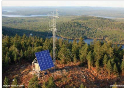
A solar array on a ridge powers a site in a remote location where an electrical grid tie-in is not available.
