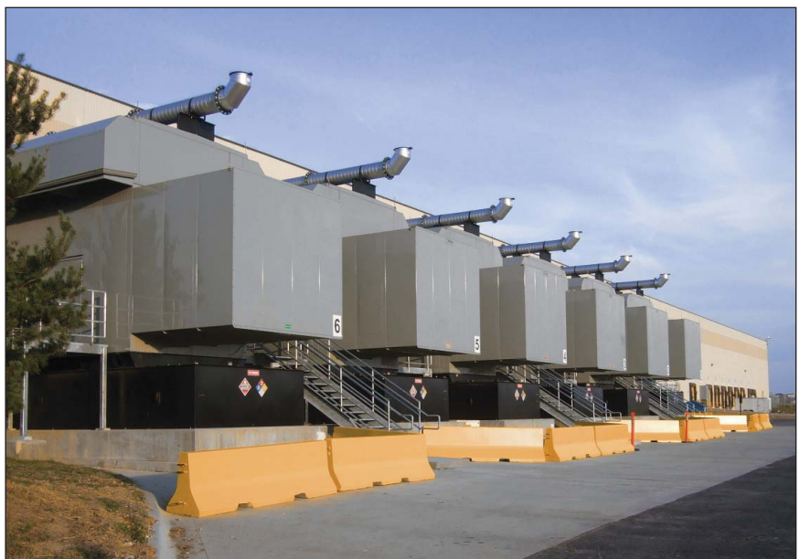
Emergency standby generator sets capable of an 85 percent average load factor have distinct advantages in critical data center applications. (Photo courtesy of MTU Onsite Energy)
