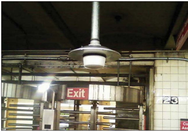
The antennas that hang from the ceiling resemble hanging lights, in effect hiding the antennas in plain sight.
