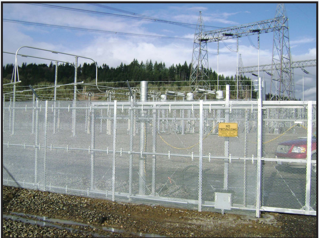
Oak Ridge National Research Laboratory experts helped install a cost-effective security system to guard a utility substation against copper thefts.
