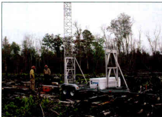
A Pepco 100-foot crank-up tower serves the emergency repeater.
