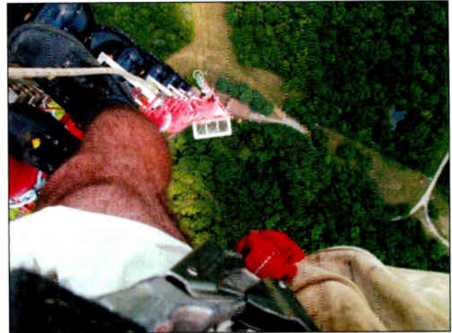
A view from the 1223-foot level on the WKDF tower in Nashville, TN. Tower hands cannot follow the advice, 'Don't look down!'
