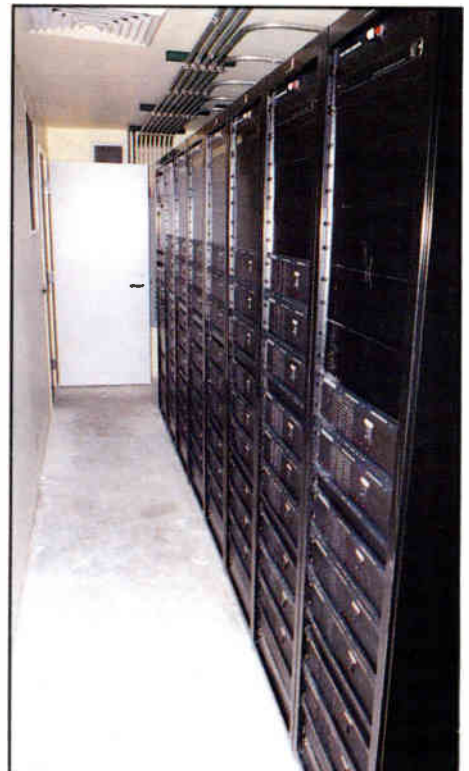
Exhibition Hall sound racks. Conduits are for AC feeds for each rack.
