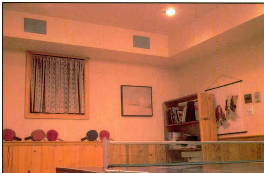
Yamaha in-wall speakers were also installed in the playroom.
