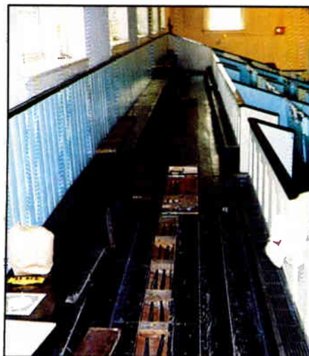
The sound-system wiring is under the balcony floorboards. Each transducer makes a home run to a junction box near the balcony.
