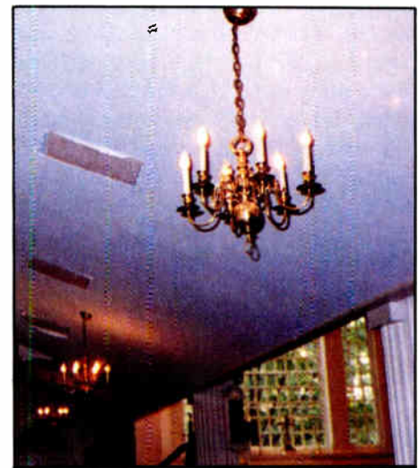
You can see where we set four panels into the under-balcony ceiling. Then we patched them with plaster, canvas and paint. If you visit the church soon and look closely, you may be able to see the panels' outlines, which will disappear with age and repainting.
