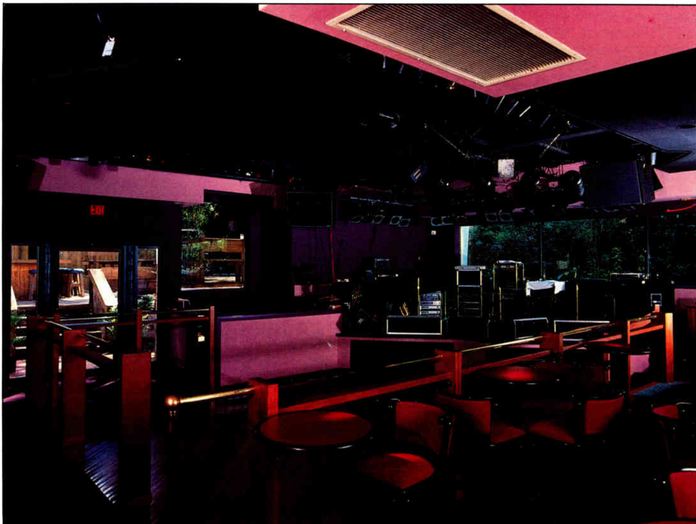
The dance floor at Mugwumps. The ceiling-suspended main speaker cabinets flank the stage; behind them are the side speakers. The rear speaker cabinets are at left, foreground and background.
