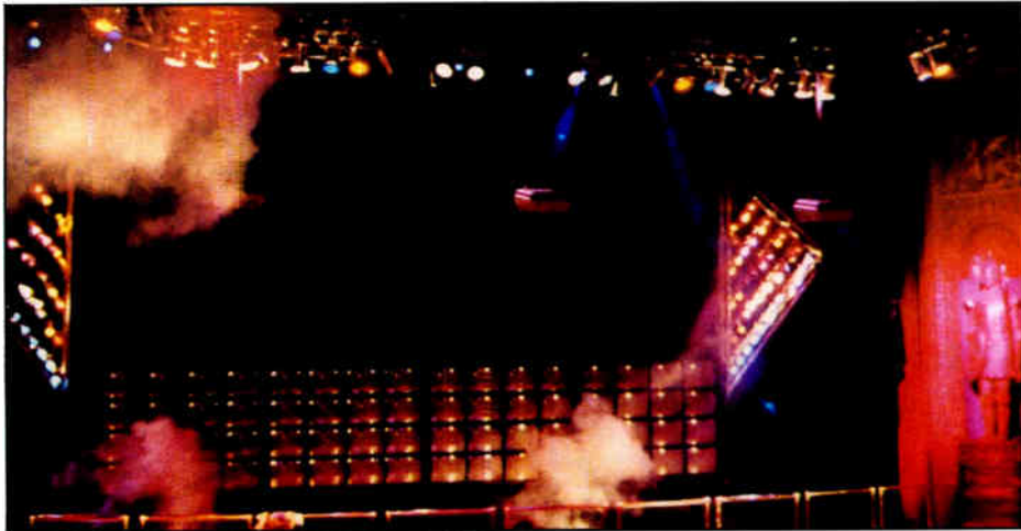
ClubLand uses the E-V MT-4 (upper left), DMT 2181 (center) and the DML-1152 for the audio for dancing.
