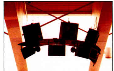
Figure 8. Front view of a completed array based on Umbulus as installed in The Church of the Risen Savior, Burnsville, MN.
