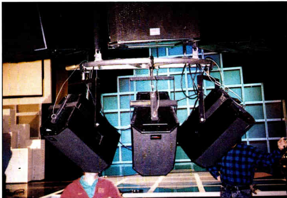
The low weight-bearing capacity of the ceiling made placement of the Apogee loudspeakers a challenge.
