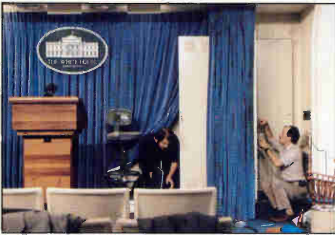
Chris Nottingham (left) and Keith Dorest of Professional Sound Industries install a sound system rack in the White House Press Lobby.
