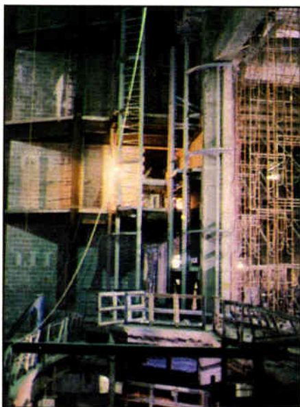
This construction shows the aluminum framing for the acoustically transparent proscenium being erected in front of the structural proscenium.
