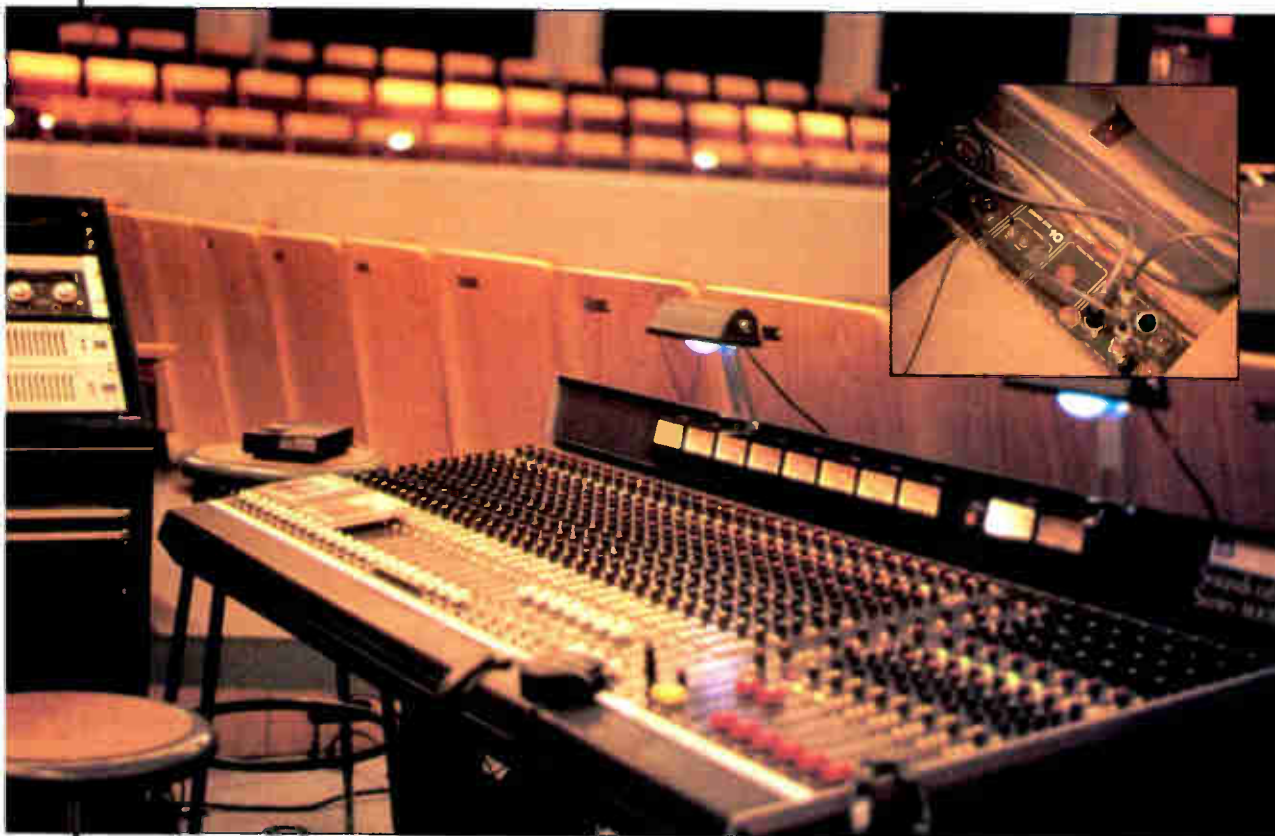
The mixing console's location on the floor; (inset) the console's patch box. A second console is located in a control booth.
