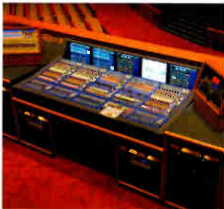
The Midas XL8, an installation at the Westover Church in Greensboro, North Carolina.
