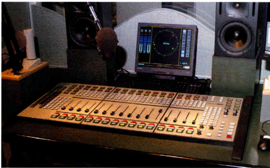
A Klotz VADIS control surface at KCRW
