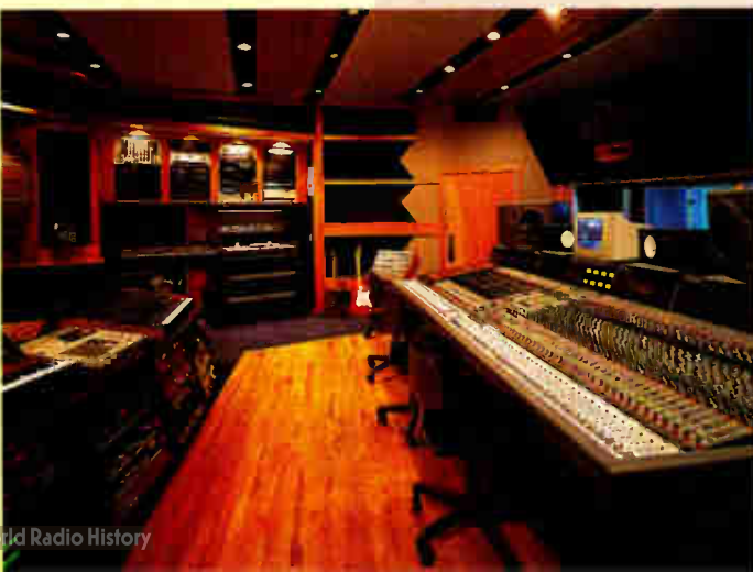
Named for its inspiring river view, the Hudson Suite of Chung King's new Varick Street Studio was completed this February. The studio was designed by owner John King and Frank Commeatale and features a 72-input Neve VRP with Flying Faders, Augspurger 215 mains, and 48 tracks of both analog and digital Studer recorders.
