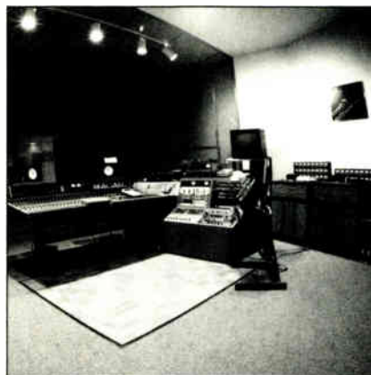
AVANCHE RECORDING STUDIOS Northglenn, CO
