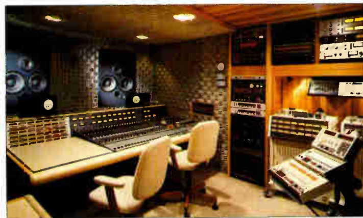
KLUB KEV'S recording co., Seattle: Scott Spain and Dr. Lloyd Cable, the operator and the engineer, designed their own main control room for KLUB KEV'S recording co. in Seattle. The front wall contains 10 inches of sand, Sonex foam and Westlake BBSM-12VS monitors, which are floating on 3-inch neoprene dowels. That's a Neve 8232: the room opened in January 1990.
