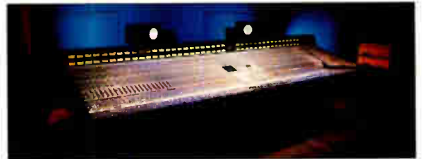
Battery Studios, NYC: The Studio A mix room with an SSL G Series console at Battery Studios, NYC. The facility, which opened in October 1989, includes three rooms in 6,000 square feet of "technical" space. A Tannoy double-15-inch monitoring system is powered by Perreaux amps. However, monitors are removable and replaceable within 20 minutes, something of a trademark for designer Russ Berger of Russ Berger Design Group, Dallas.
