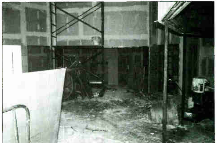
The two in-construction views are from Russ Berger's (of Dallas-based Joiner, Pelton & Rose) LEDE design for Otis Connor's new Studio Centre, which is due to be completed this month. The back wall of the large control room was fitted with twelve RPG quadratic residue diffusors. The top photo is taken from the rear of the control room looking outward over the mixing position. The lower shot shows the drum booth (in background, behind scaffolding) and some detailing of the control room front wall construction (upper right corner of photo). Compare these to the studio's floor plan, printed on page 90.
