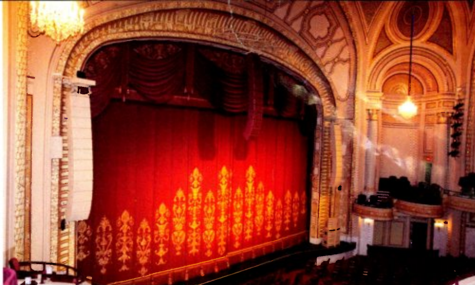
Palace Theatre's installation of a Nexo GEO S12 system
