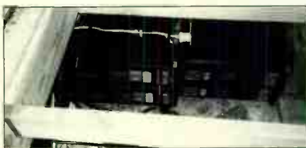
Three IT-1220's paired with three AR-1220 Voltage Regulators visible under the floor at Vital Recording.
