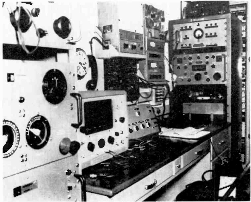
General view of control desk of typical U. S. Army ground station, with main control panel (inclined) at right-center. Satellite-to-ground receivers are in cabinet at far right. At left is the remote control equipment for orienting the antenna.
