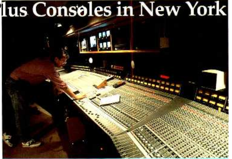
▲ SL 4080 G Plus console installed at CBS's Ed Sullivan Theater, New York
