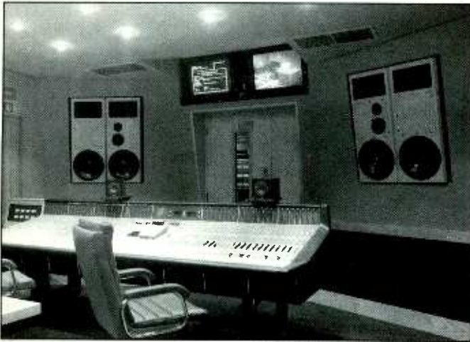
The BB5 XBD system installed at BBC Maida Vale London
