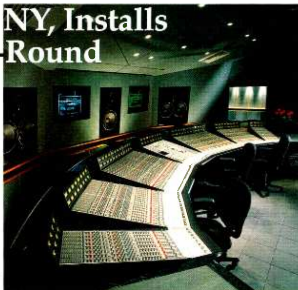
▲ Customised, crescent-shaped SL 4000 G Series console, with additional custom-built furniture, installed in Studio 4 at The Hit Factory Digital Recording Studios, New York City
