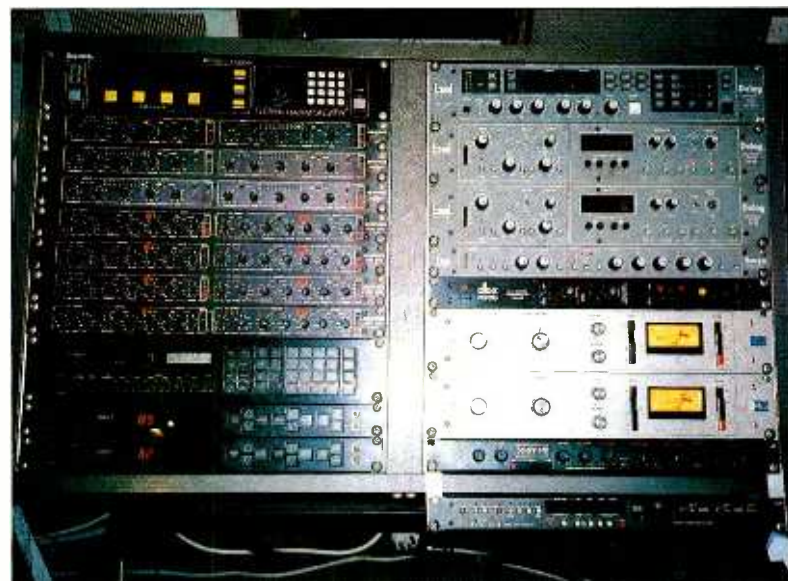
Outboard equipment rack
