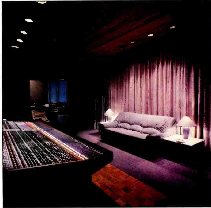
Rear of main control room
