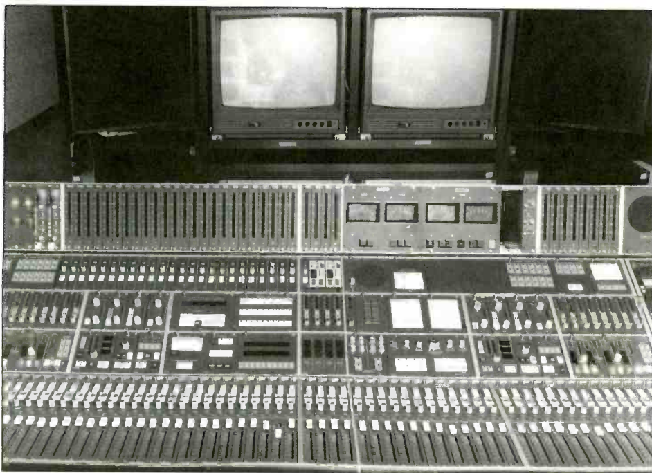
Digitally assignable Calrec console installed in BBC Master sound control vehicle.
