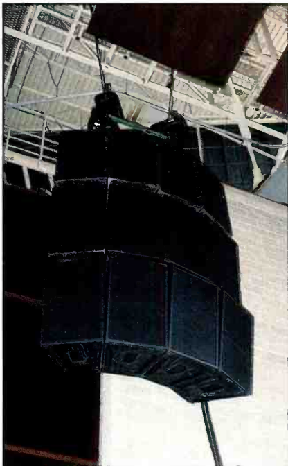
EAW KF850 enclosures are suspended in a hanging array. One dozen cabinets are hung from Sun Sound's custom aluminum fly bar with two chain motors.
