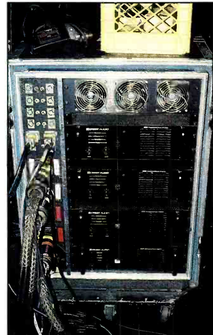
Each of Sun Sound's custom power amplifier racks house four Crest 8001 power amplifiers. Input and output signal cables are connected on the front panel.
