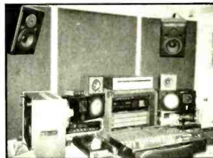
Mixing and recording hardware at Musitech includes a Soundcraft series 200 console, Otari MX-5050B 8- and 2-tracks, and Electro-Voice Sentry 100A monitors.
