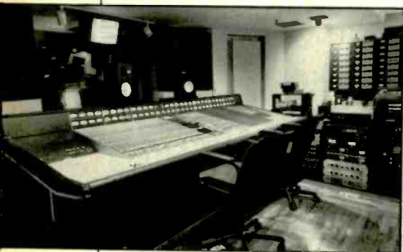
39th Street: SSL 4000E installation.
