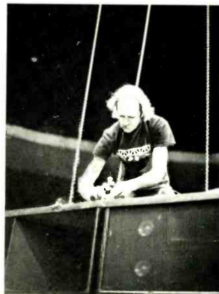
Figure 5: Half-inch bolts are used to secure the upper metal frames and truss bars together. (Shown: audio crew chief John "J.T." Taylor.)
