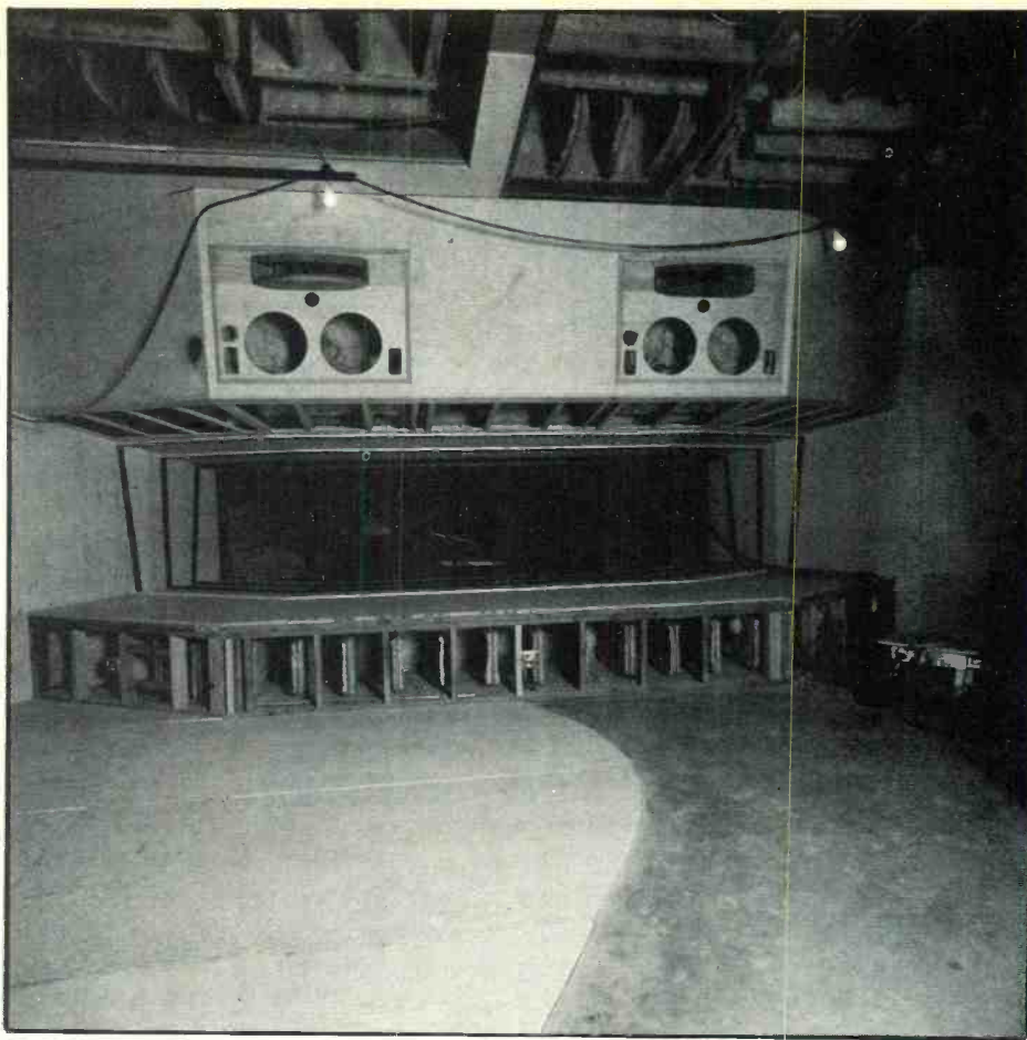
construction detail: split slab, ceiling traps, monitor framing, looking toward control room window
