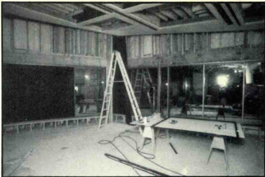
construction view: showing sliding mirror wall installed in front of acoustic trapping system
