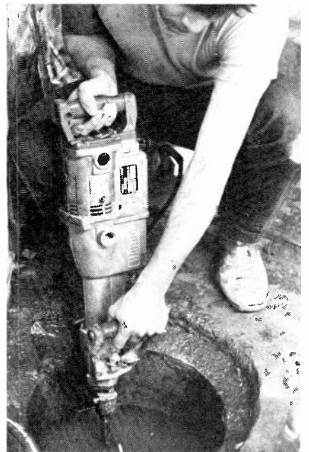
In the beginning: sanding the walls, putting in insulation, digging out the sump pump
