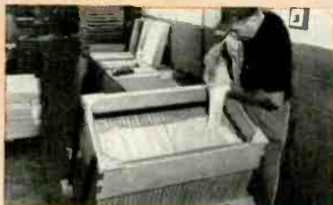
3. Sand is poured on, filtering slowly through small openings into panel cavities. Vibration machine eliminates air pockets, insures maximum compression.
