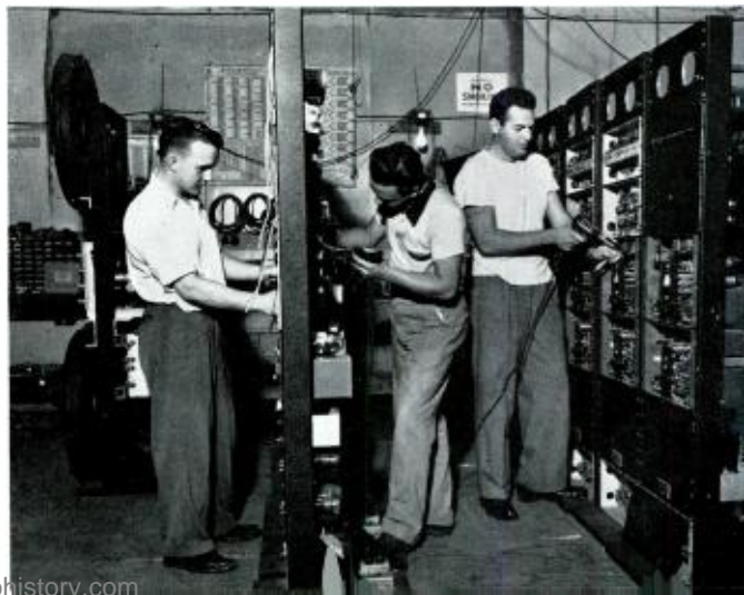
Technicians assemble and wire control-equipment at the Oyster Bay station. Cinerama records on seven separate sound channels.
